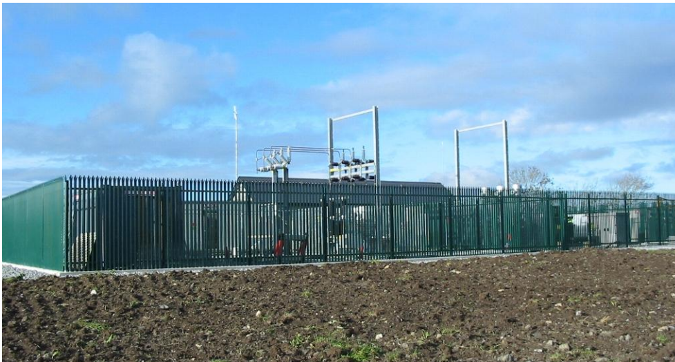
Figure 2-23 Typical Substation Compound
